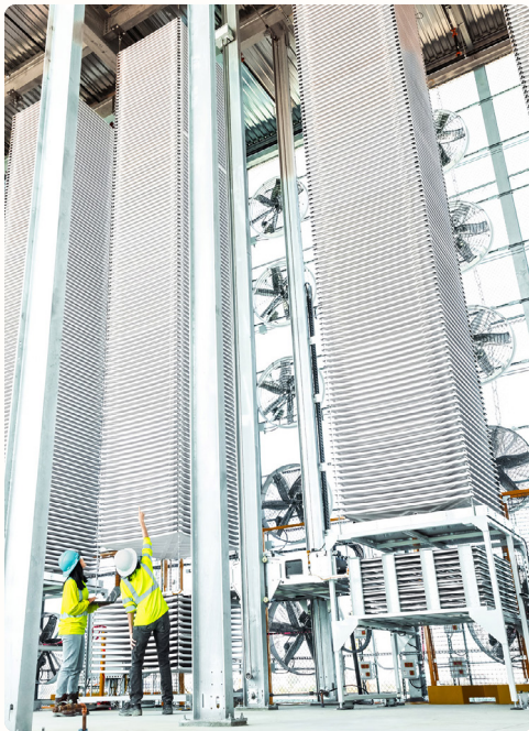
BEV portfolio company Heirloom's Direct Air Capture facility
